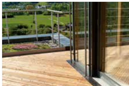
The design of thresholds is flexible as long as they correspond to the "Flat Roof Guidelines" or any relevant national regulations.
